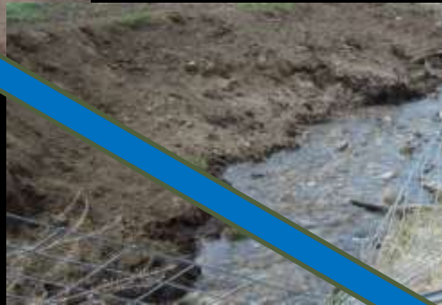
Eroding stream banks Contributing 300 kg/yr
